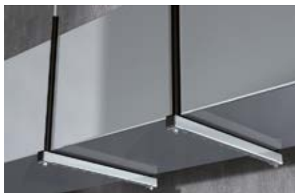
Airduct with Hangszigetelés on installation channel
